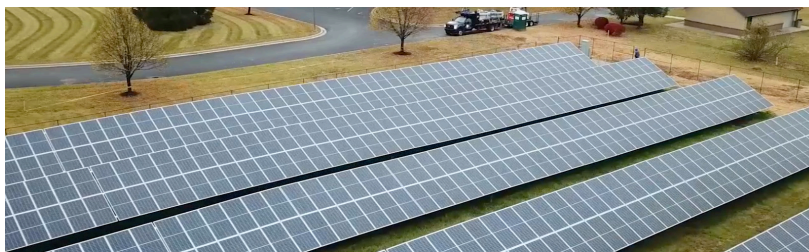
Four Noblesville Schools properties are currently producing energy provided by the sun for the school corporation's use.
